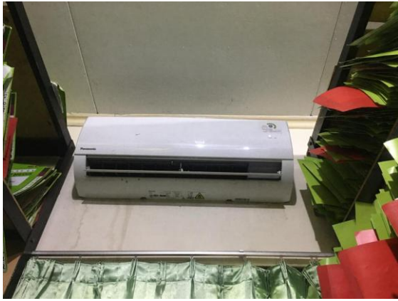
AC (Air Conditioner)
