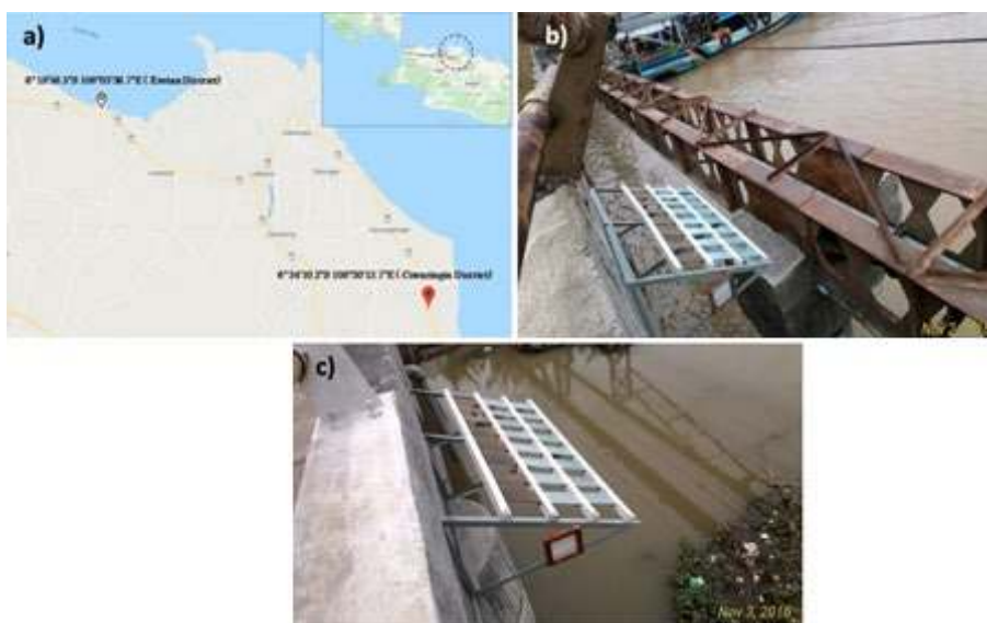
Fig 1. (a) Location of two field sites in West Java Province; test racks of atmospheric corrosion in (b) Eretan District and (c) Ciwaringin District
