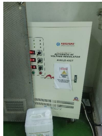
Gambar 16. Regulator listrik area dapur
